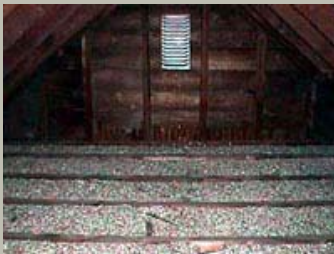
Vermiculite insulation found in an attic.
